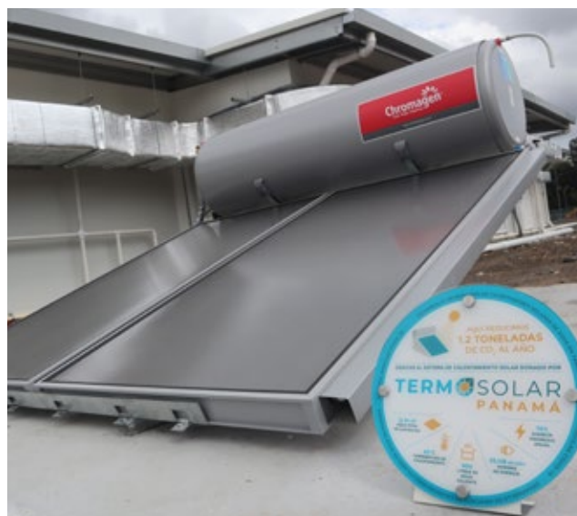
Installation of a solar water heating system at the Panama Solidario hospital in Panama City. Photo: Termosolar - UNEP.
