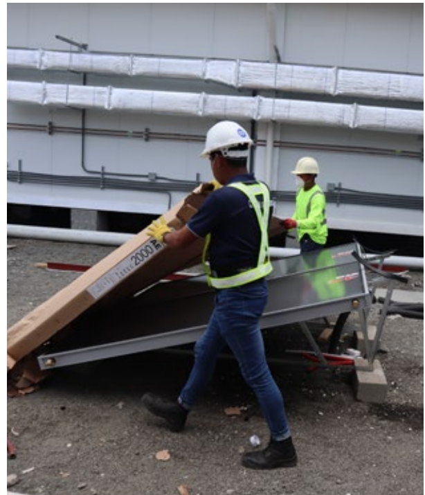
Installation of a solar water heating system at the Panama Solidario hospital in Panama City. Photo: Termosolar - UNEP.
